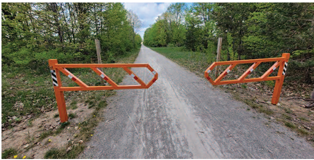
A set of previously installed gates, similar to what will be installed along the North Central State Trail in Otsego County. (courtesy of DNR)
